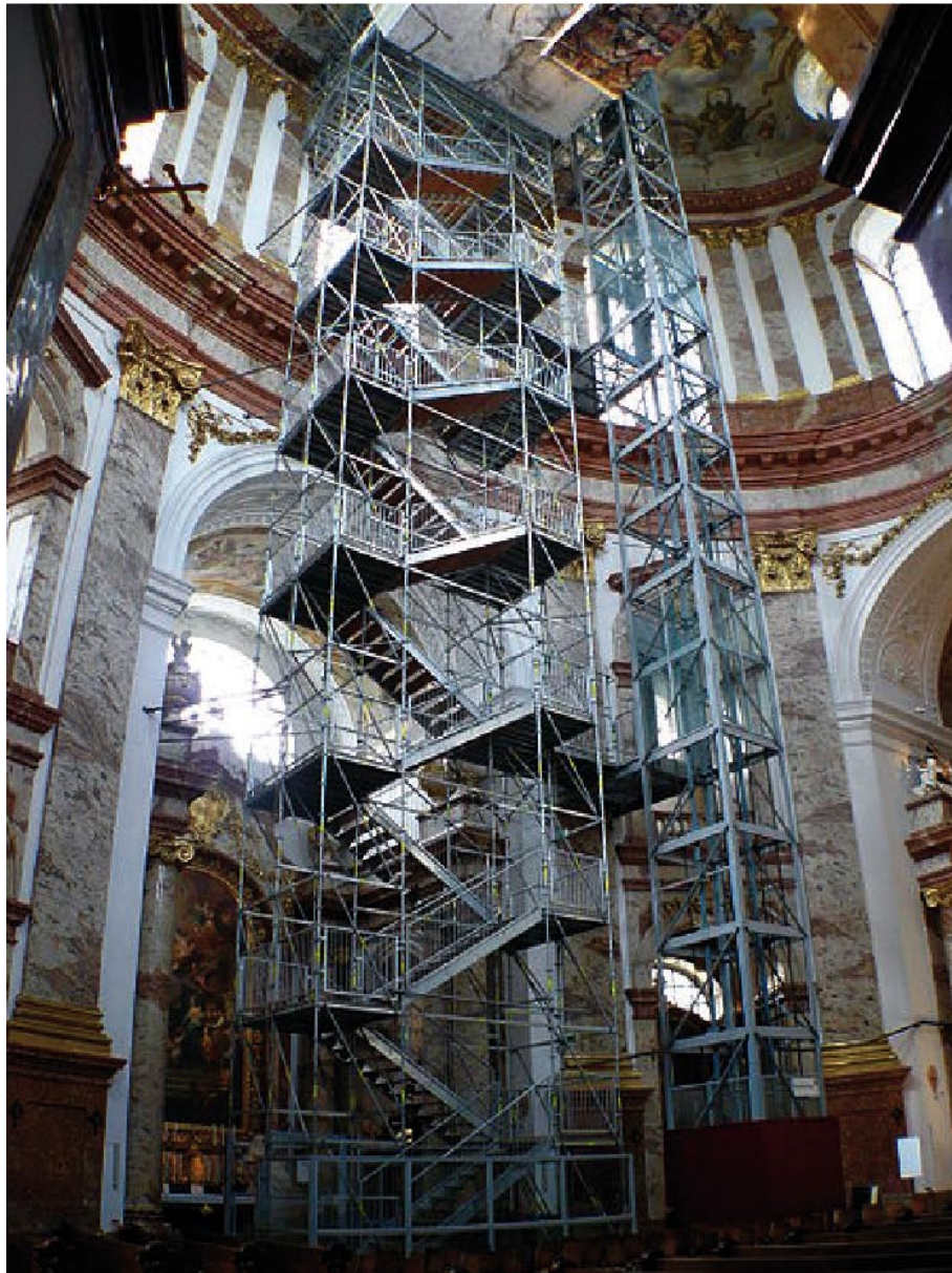
PHOTO 2. PASSIVE-INTERACTIVE PARTICIPATION : KARLSKIRCHE IN VIENNA, AUSTRIA, 1716-1737 (INTERNAL TEMPORARY LIFT AND VISITORS' PLATFORM).
