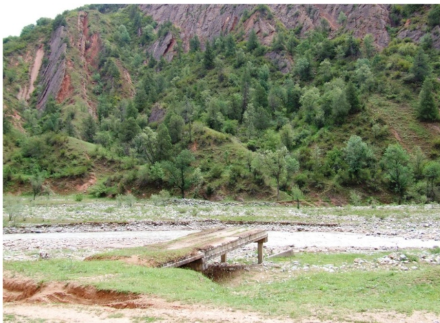
Fig. 11 Broken bridge (not) crossing the Otuz Art River. During Soviet Times, several bridges over the strong and swift river were erected and maintained by the collective farms. Nowadays, most of these bridges are broken. Every year several people and many animals lose their lives. In 2014, the reconstruction of the bridges was still pending since it was a cost-intensive investment that had to be done mainly by the users themselves. Photograph: author
