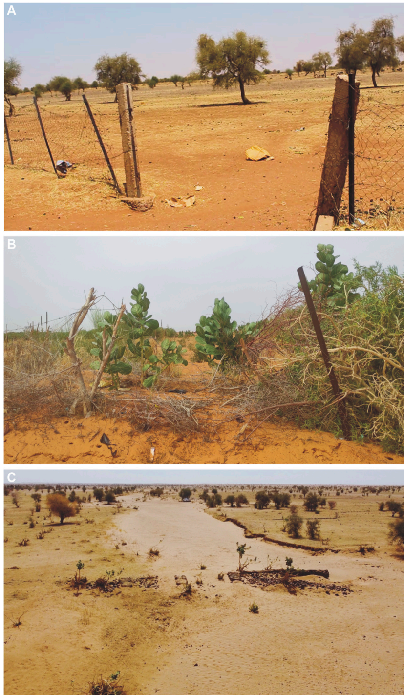
FIGURE 11 | Examples of deteriorated infrastructure. Two examples of broken fencing: (A) entrance to the restored plot of the Save the Children project in Monguel (Gorgol) showing the damages to the fencing and passageways without an access gate and (B) broken fence reflecting the need for fence maintenance in Bassikounou. (C) Aerial image of a damaged gabion after an important flooding event in the floodplain of Gorgol (original photos by M. Veitez-García).
